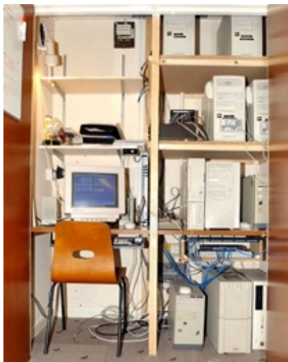
The Myriad servers installed in the IT Cupboard.
